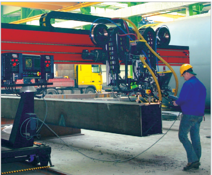
Welding process START/STOP available from one C&B control operating panel.
